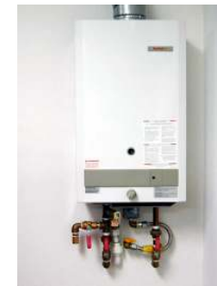
Hot water production
